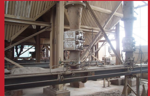
Pollution Control Valves in energy plant increased production by 10%, reduced emissions and maintenance costs.
